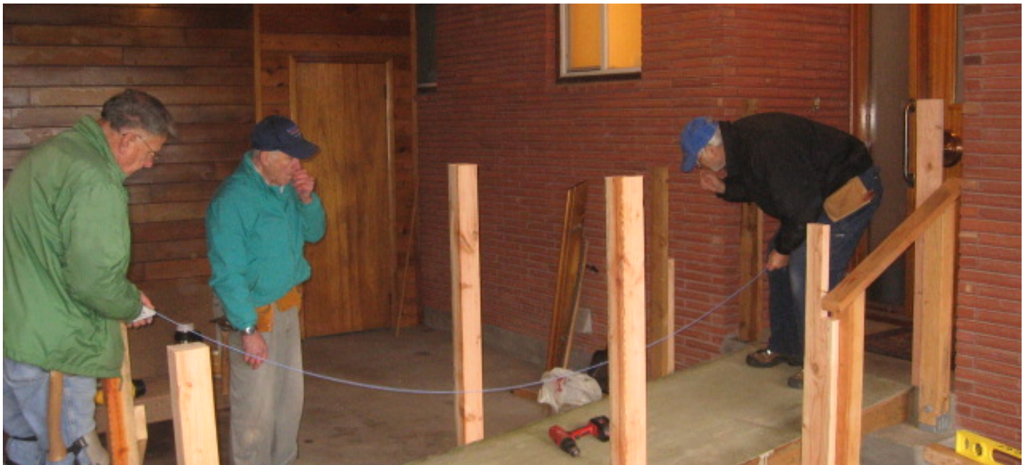
Ramp in place and posts installed. Jack Hawker and Mike Graham use a chalk line to establish the height to cut off the posts for the top railing.
