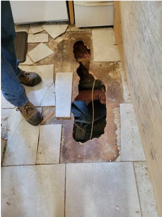
Lot A – before repairs
